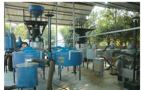
250 kW biomass gasification based power plant
