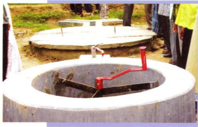
A biogas plant financed by IDCOL
