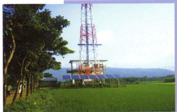
Solar-diesel hybrid power system for BTS of Grameenphone Ltd.
