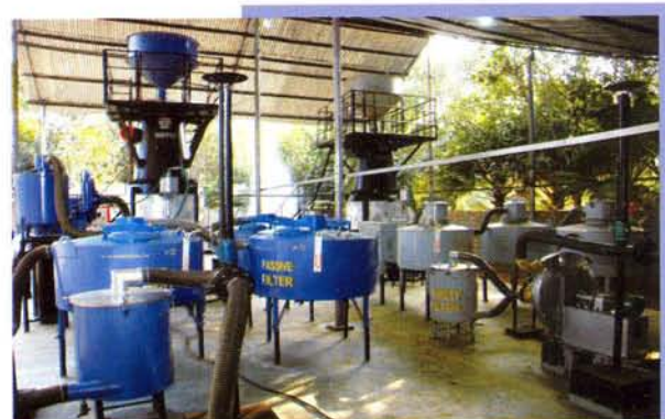
400kW biomass gasification based power plant
