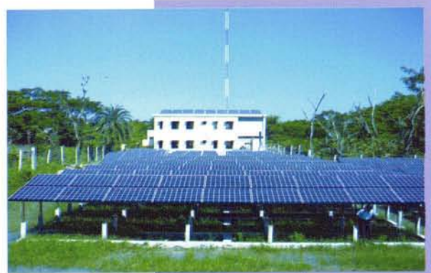
100 kW Solar PV based mini grid at Sandwip
