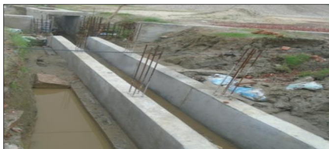
Photo 3.2: Storm water drainage system
