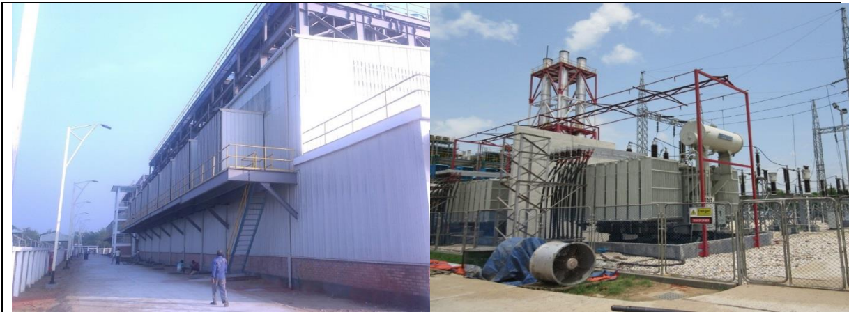
Photograph: External view of the plant (partial view and transformer)
