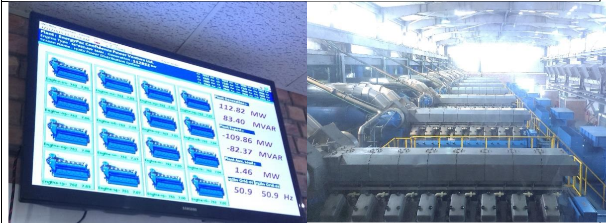
Photograph: Internal view of the Plant (production record and gen sets)
