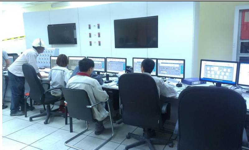
Photograph: Control monitor
