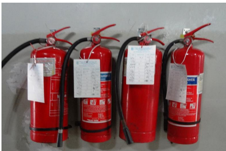
Figure 8.2: Fire Safety Equipment
