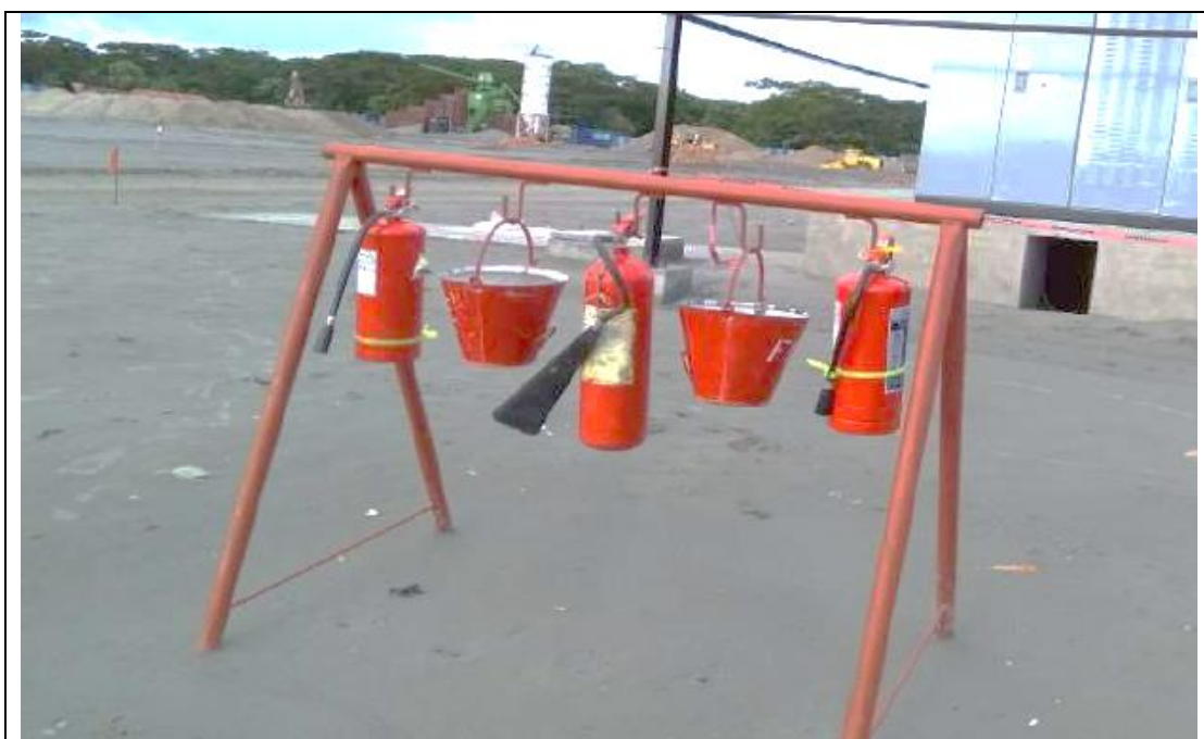
Photograph: Fire-fighting arrangement
