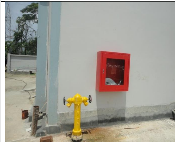
Photograph: External fire-fighting arrangement
