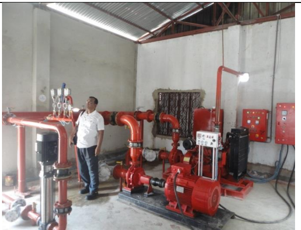
Photograph: Three pumps for fire fighting
