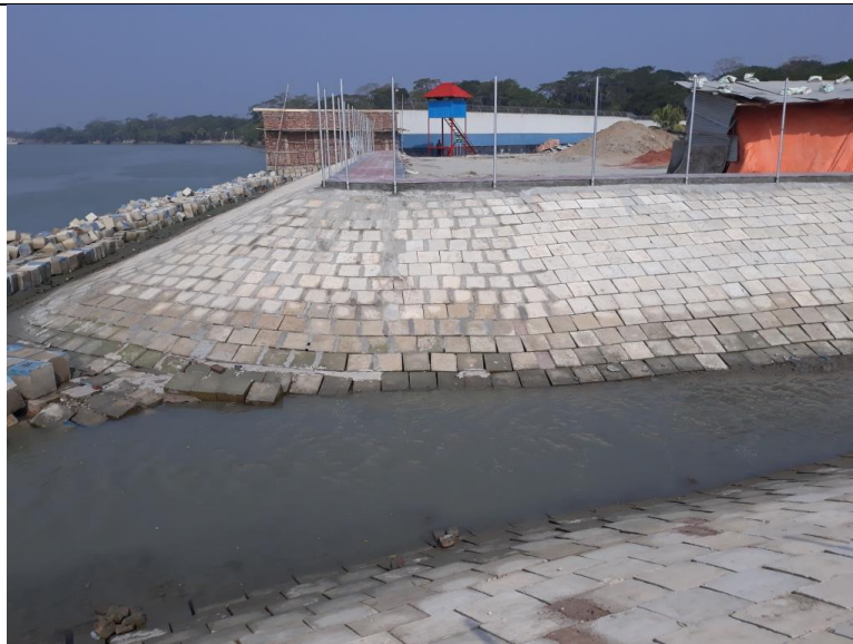
Photographs: Embankment protection arrangement
