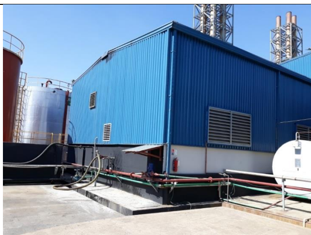
Photographs: Transformer and some important installations
