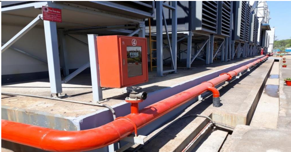
Photograph: Fire-fighting arrangement
