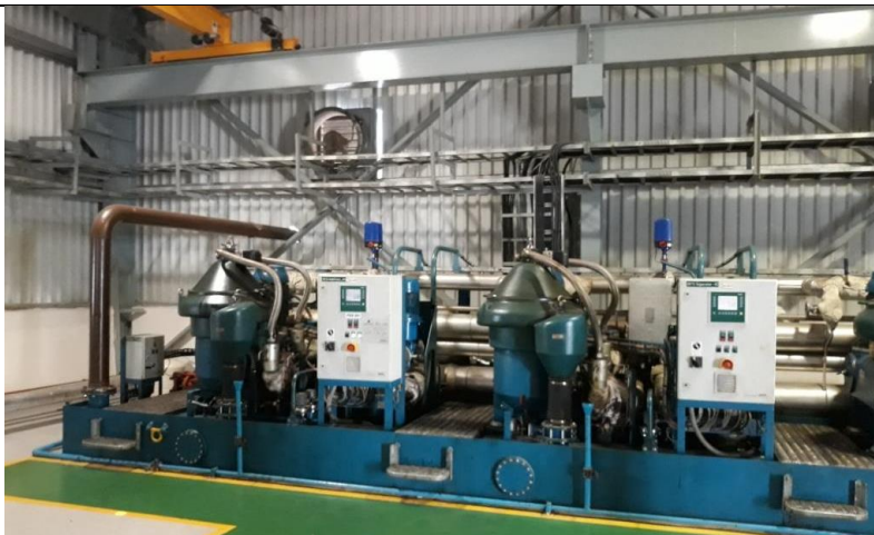
Photographs: Control room, generators and fuel treatment plant
