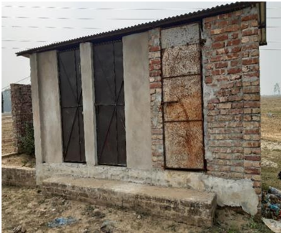
Photograph 9 (b): Toilet and Cleaning Facilities
