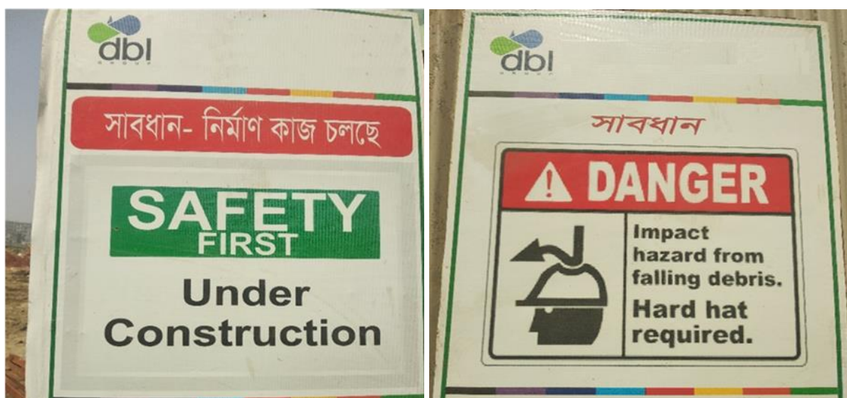
Photograph 7: Safety Signage on the site
