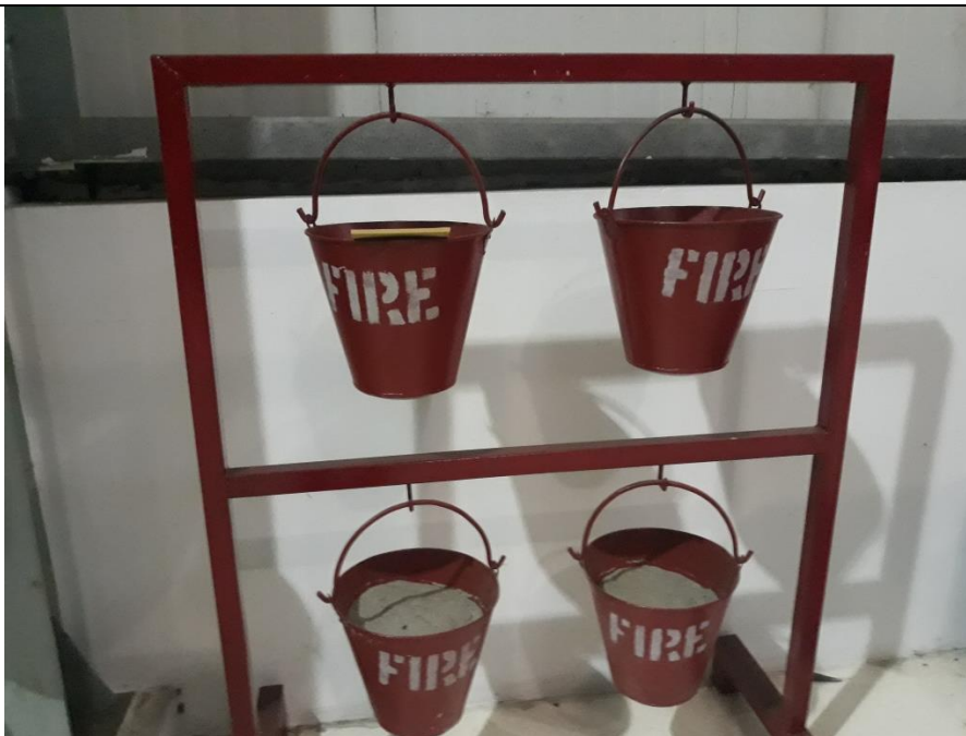
Photograph: Different types of fire-fighting arrangement
