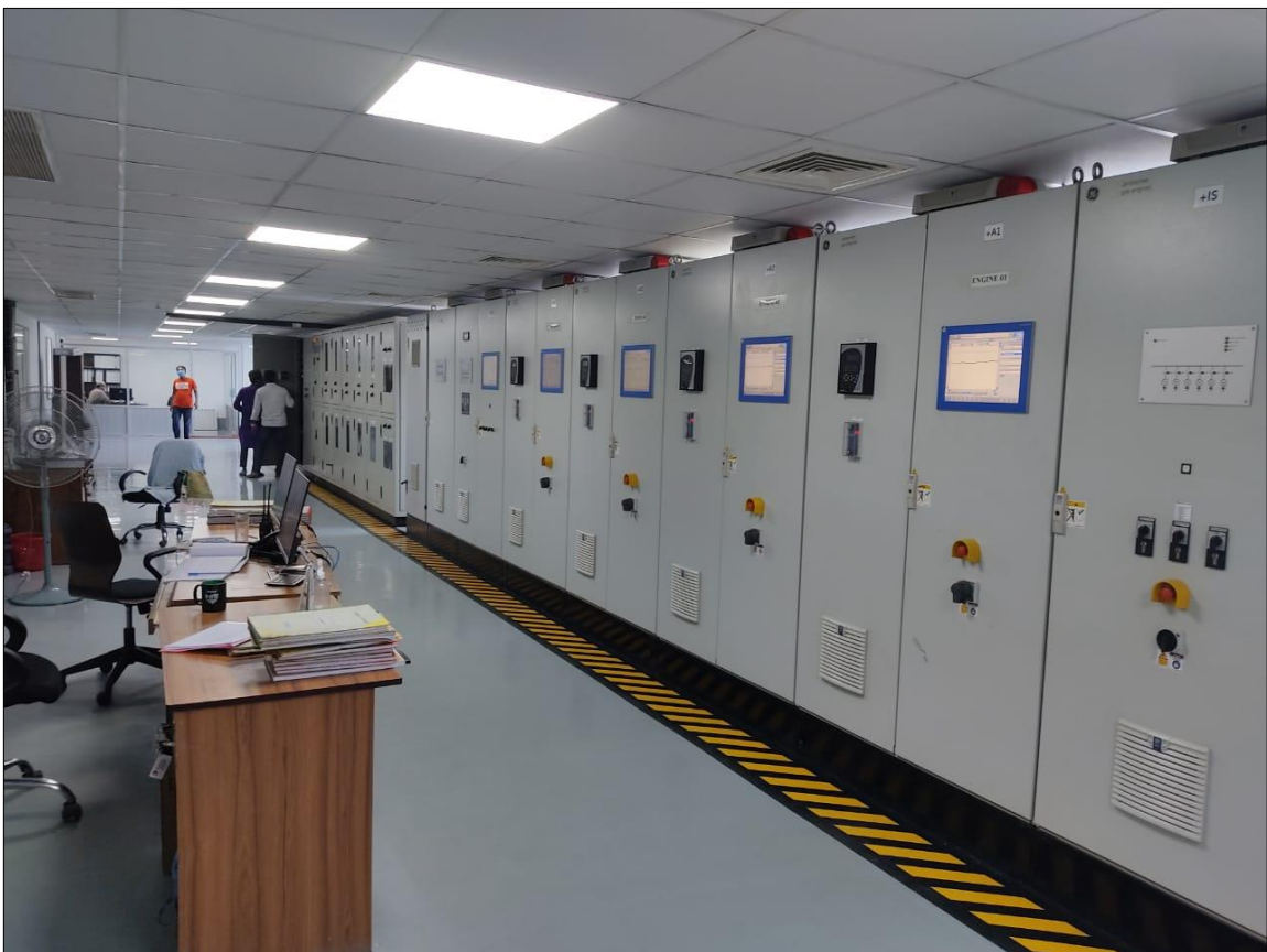
Figure 3-4: PCB (Power Control Board)
