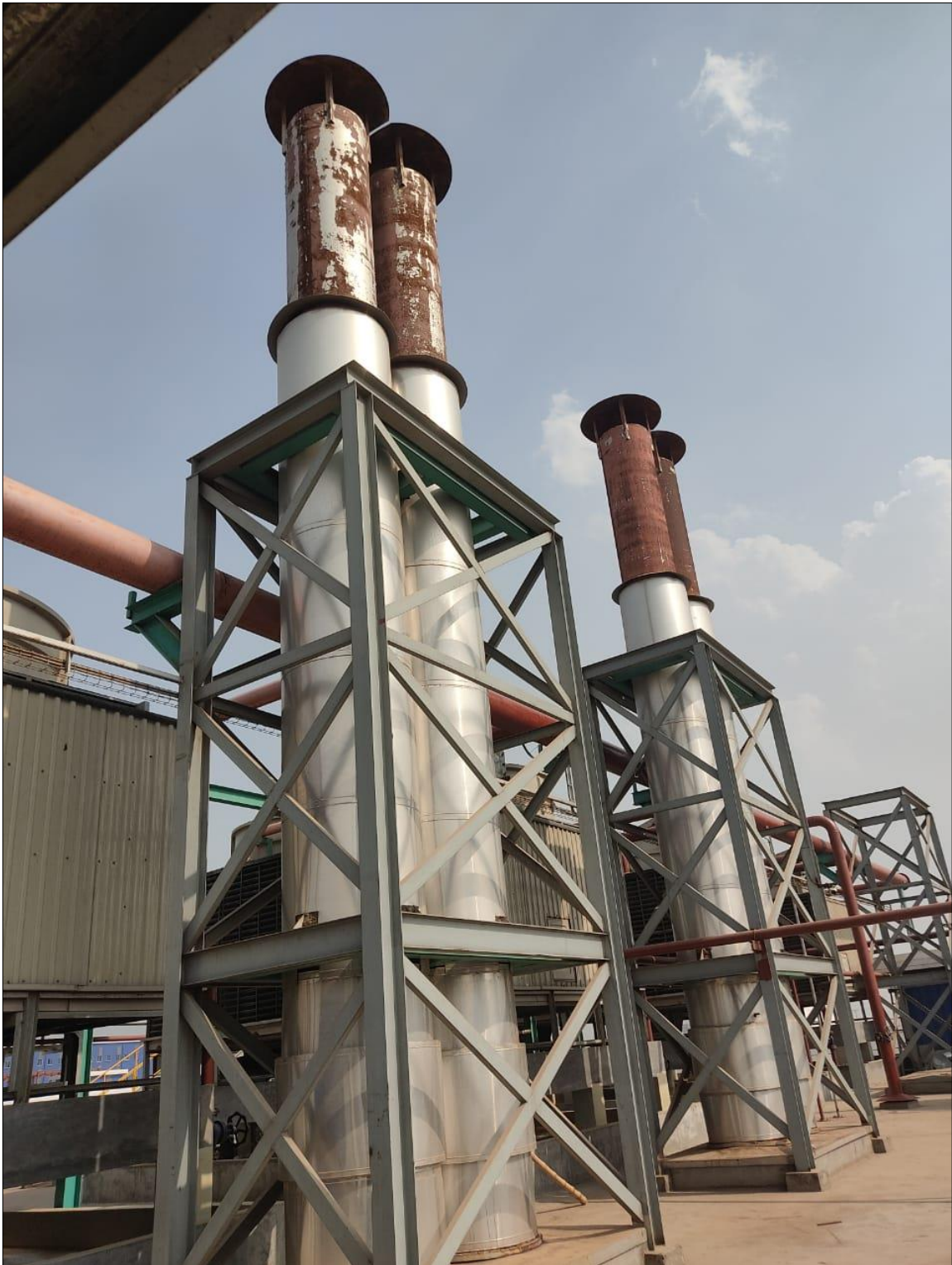
Figure 3-6: Exhaust Gas Release through this stack (stack height 39m)
