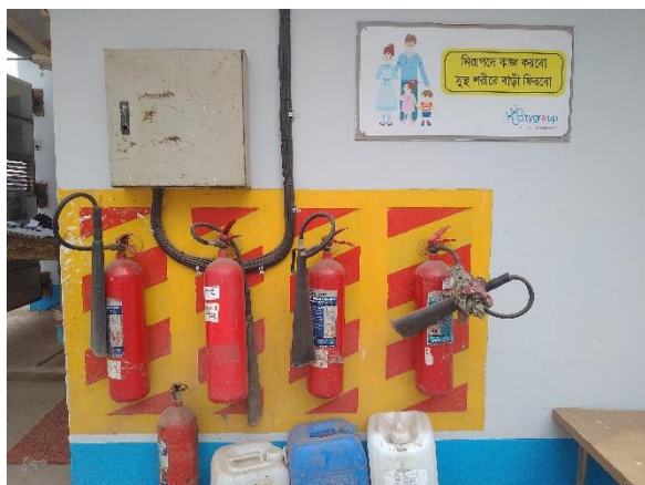
Photograph: Fire Extinguisher
