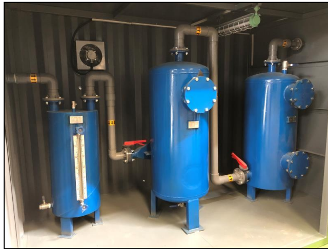
Figure 3.5: Biogas Purification Unit
